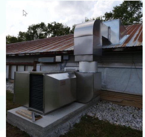
Hoosier Energy (Indiana) – Poultry barn heat recovery
